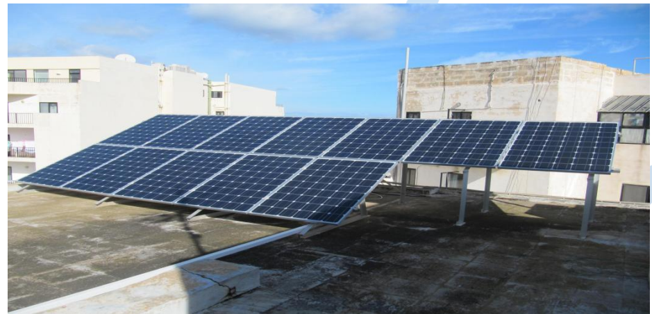
Energy Aid Scheme – Photovoltaic panels installed at roof level
